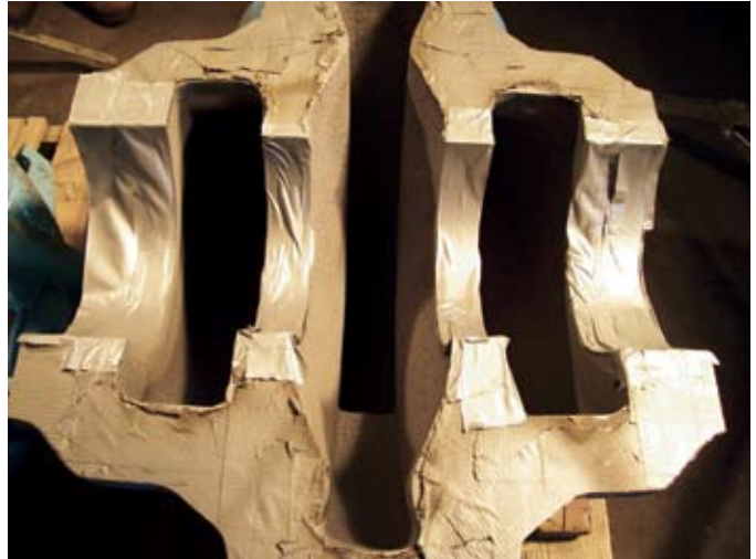
Figure 6. Denise No. 2 horizontal split-case pump – upper half of pump housing after masking the seal areas and grit blast cleaning.
