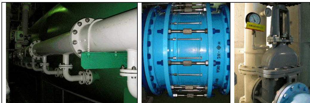
Picture 12: Polyamide coated parts in the SWRO Chatan desalination plant
