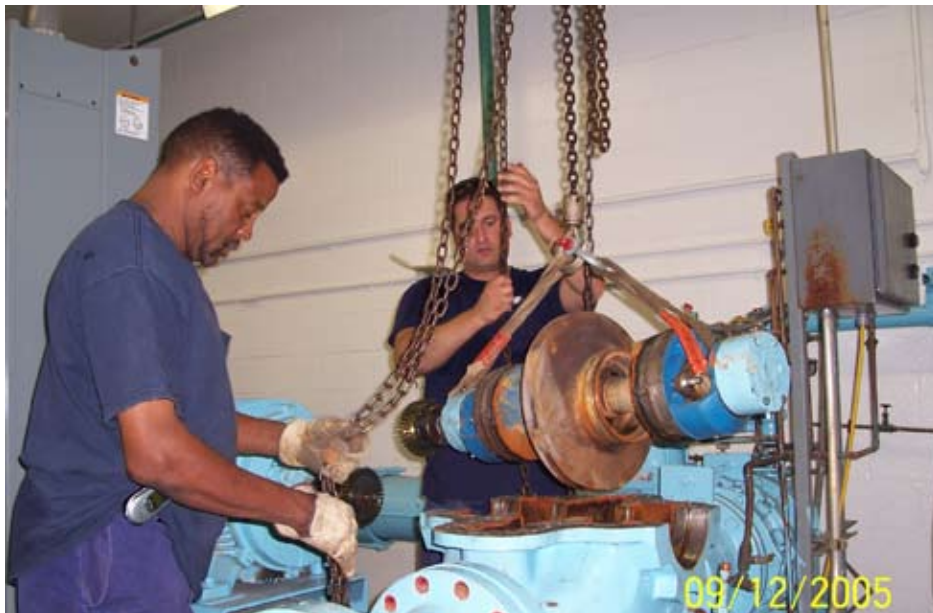
Figure 1. Denise No. 2 horizontal split-case pump being taken out of service for repair and coating.
